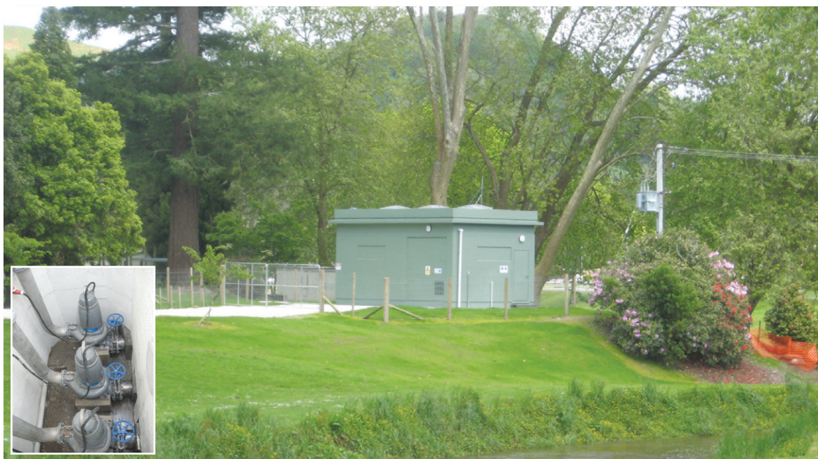
Te Kuiti Pump Station
